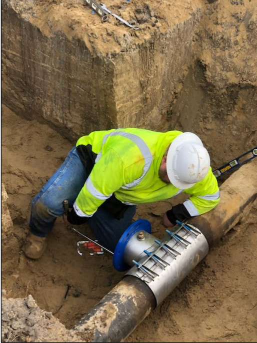
INSTALLATION OF A TAPPING SLEEVE FOR AN 8" FIRE SERVICE ON CONDOR DRIVE.
