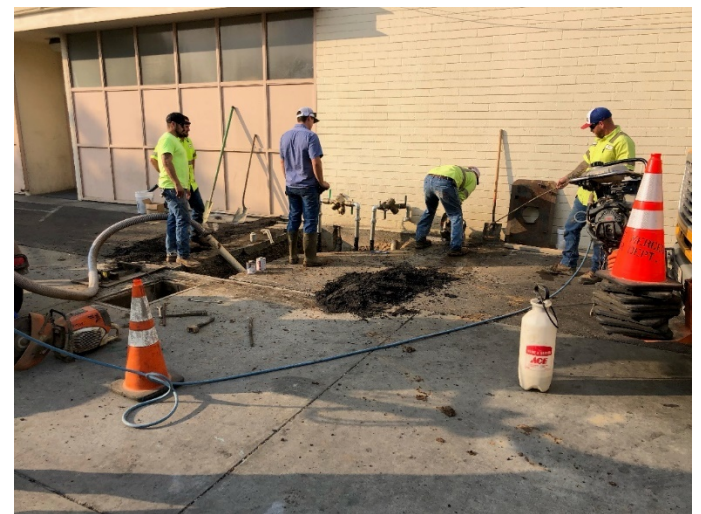
Public Works Water Crews installed a backflow at the Merced Police Central Station.
