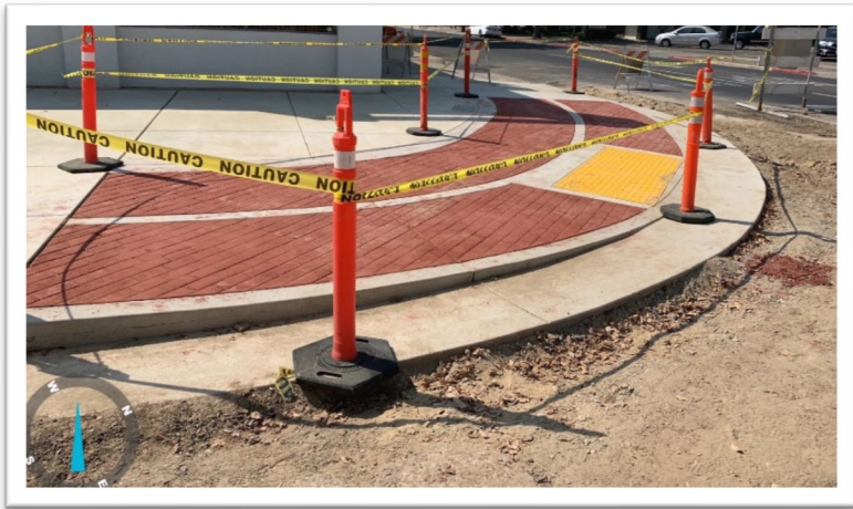
Project #120060 – N St. Improvements – 16 th St. to 18 th St. TBS Contractors, Inc. The crew poured stamped concrete. This project is approximately 80% complete.
