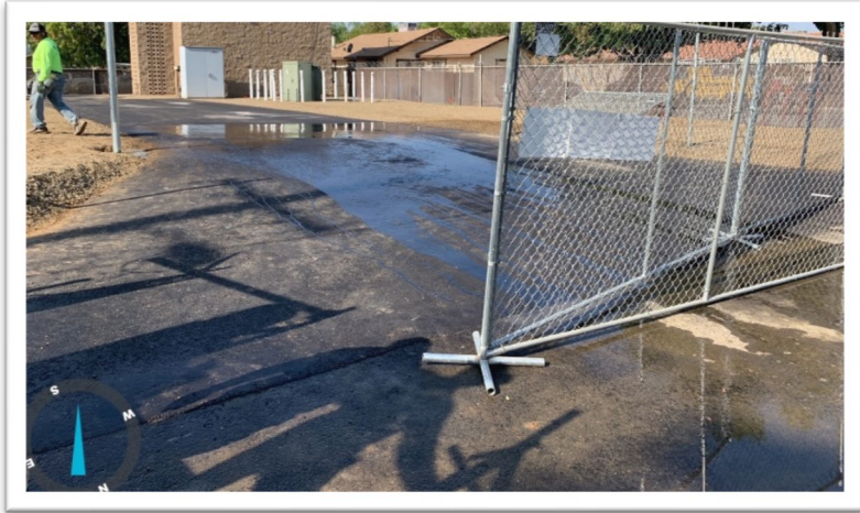
Project #117047 – G St. – Well Site 3 Tank Removal Standard Demolition Crew installed new fence and gate. This project is approximately 96% complete.
