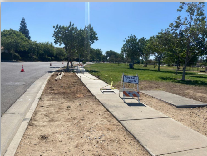
The City hired contractor is continuing work to replace sections of damaged sidewalk in the Davenport Maintenance District; this week crews poured cement.
