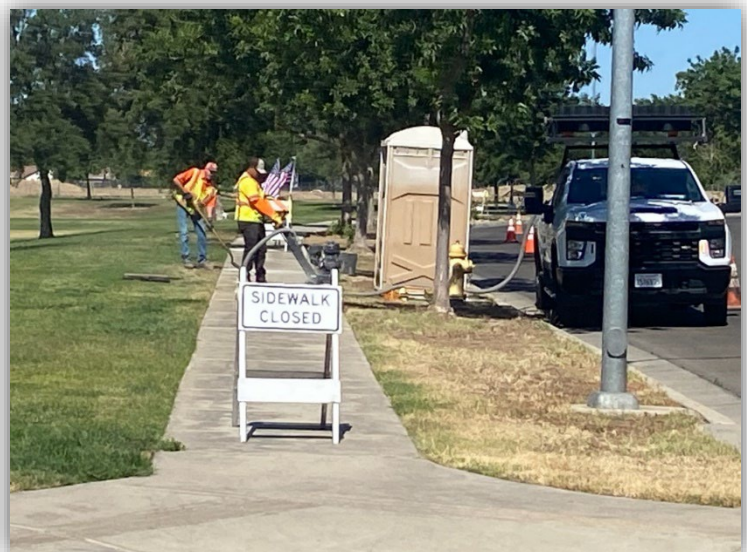
City Streets crews grinded various sidewalk locations that were not slated for replacement.
