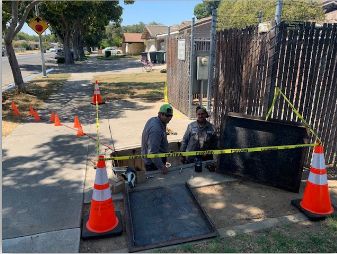
Sewer/Storm Drain Maintenance Electricians replaced two storm discharge check valves on Lopez Ave.
