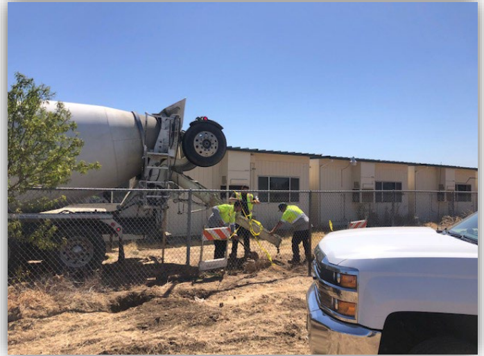
Sewer/Storm Crew poured new manhole collars near Alfarata Blvd. and Gerard Ave.
