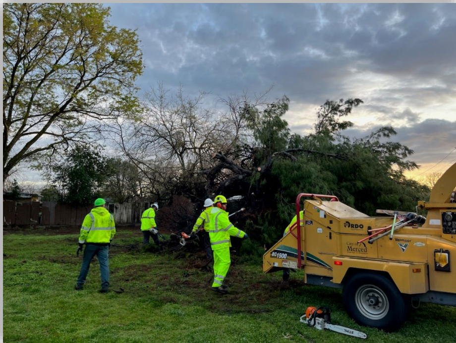
Crews removed a downed tree at Diego Rivera Park after the recent storms.
