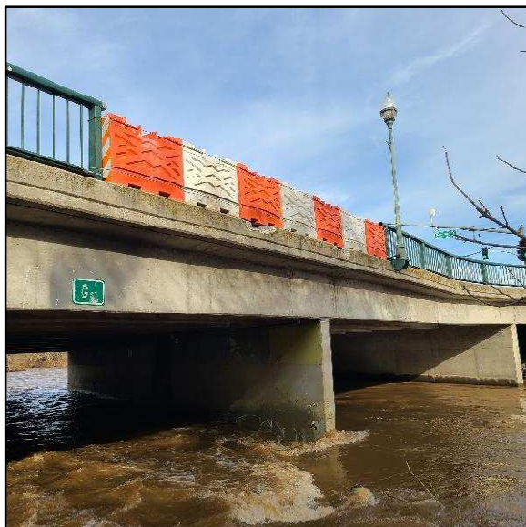
Figure 1: Elevation View of Damaged Railing (Looking West)
