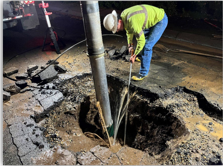
Crews repaired an 8" water main line at the 2100 block of Arden Lane
