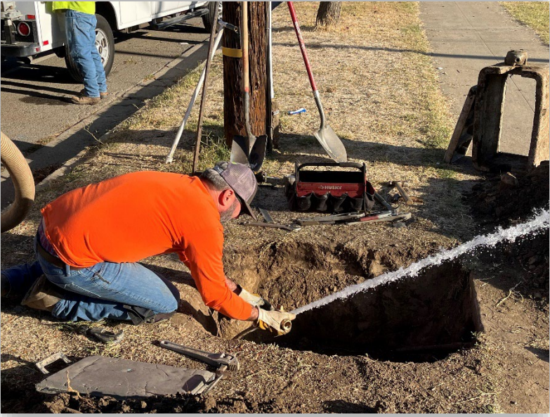
Crews replaced a broken ¾" shut off valve at the 300 block of R Street.
