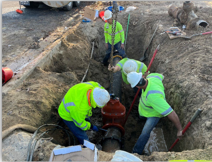
Crews replaced a broken section of an old water main line and a leaking valve on Buckner Road
