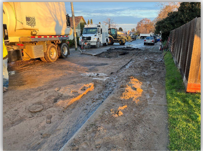
Water crews responded to an emergency water main line break near Almond & Merced Avenues
