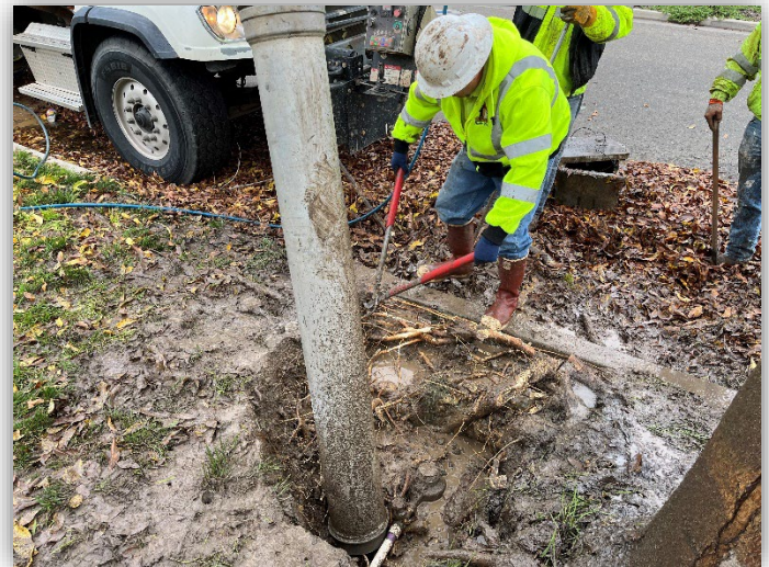
Water service was repaired due to tree root damage on Daffodil Drive
