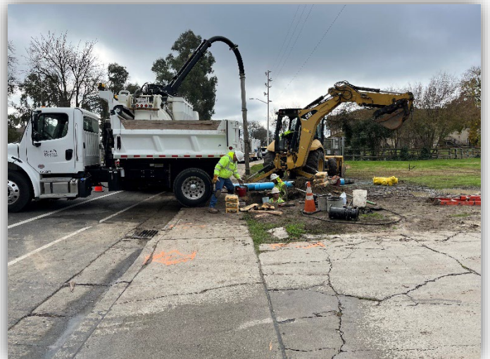
A vehicle damaged fire hydrant was replaced on the 3300 block of M Street.
