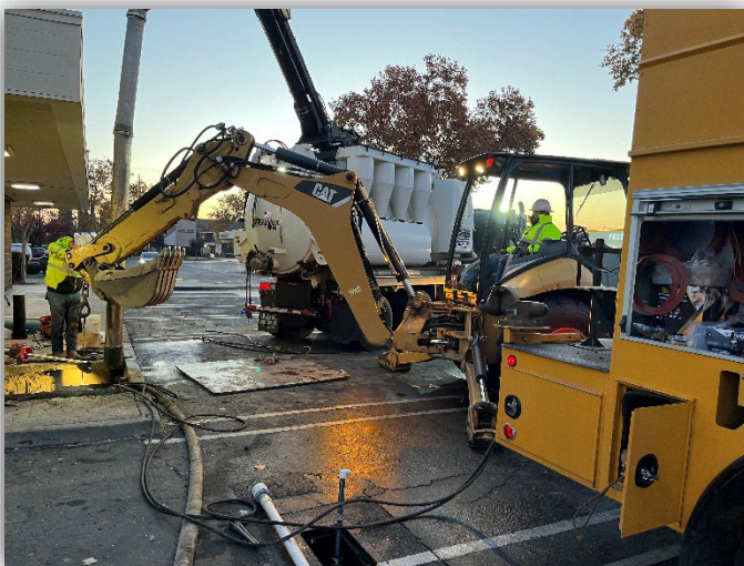
Crews worked with a private contractor on improvements to a commercial building's fire service line, located on G Street
