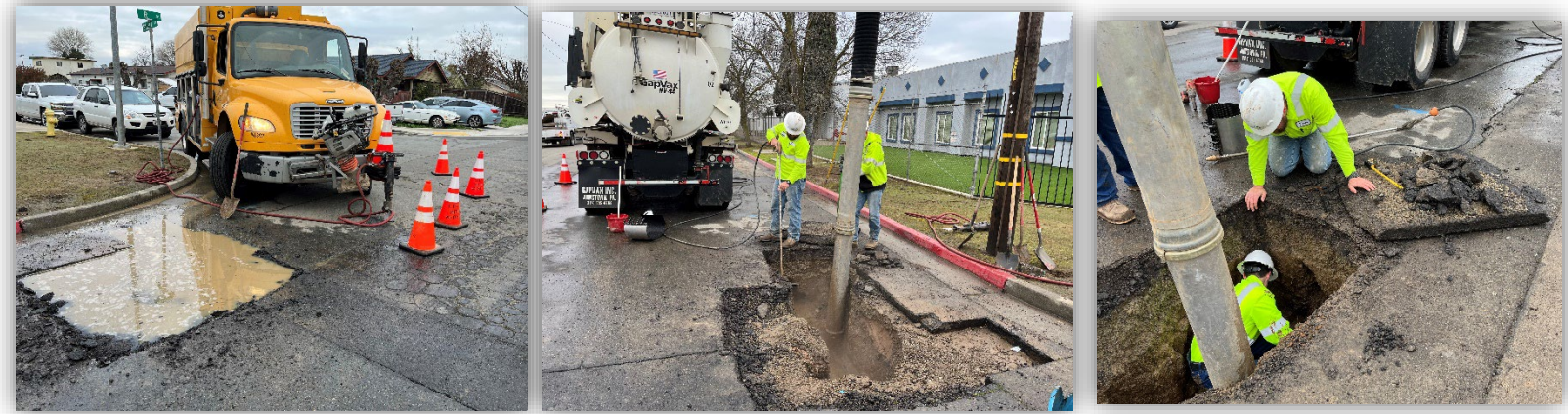
Water department repaired a water main line break at South R Street & Stuart Dr.
