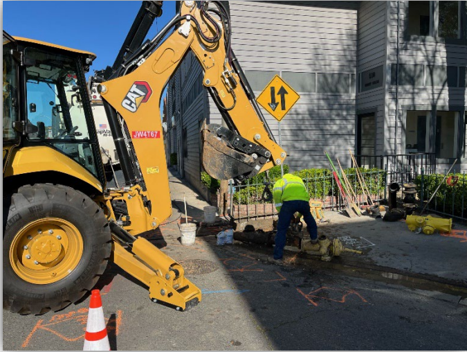
Water Department crews replaced a fire hydrant on Canal St & Main St.
