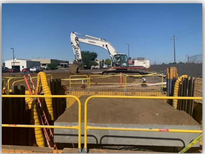
Crews chipped the outer layer of the sewer tanks inside the headworks.
