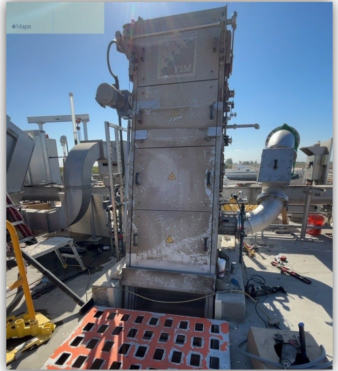
Wastewater Treatment Plant: Crews set the second screen on top of the head works. Coating the first wet well is almost complete.
