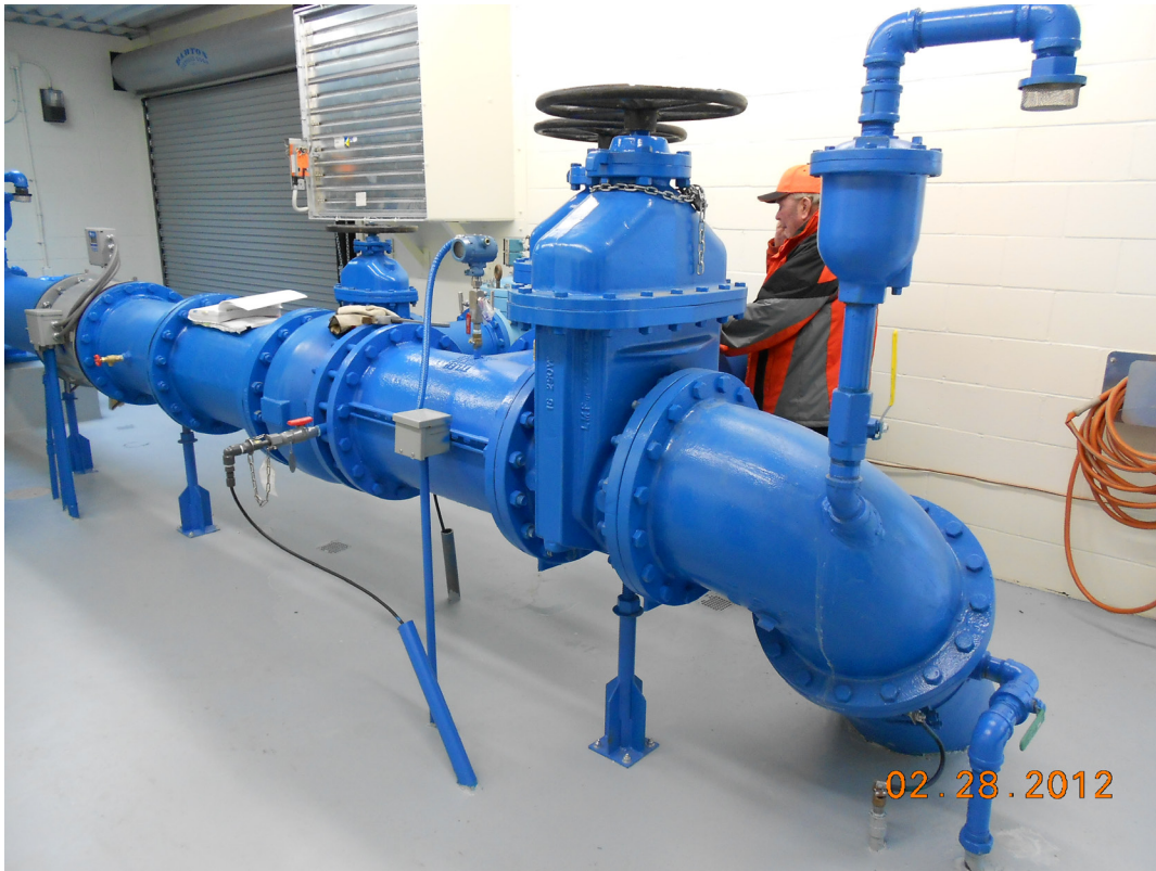
Typical pump and valve
