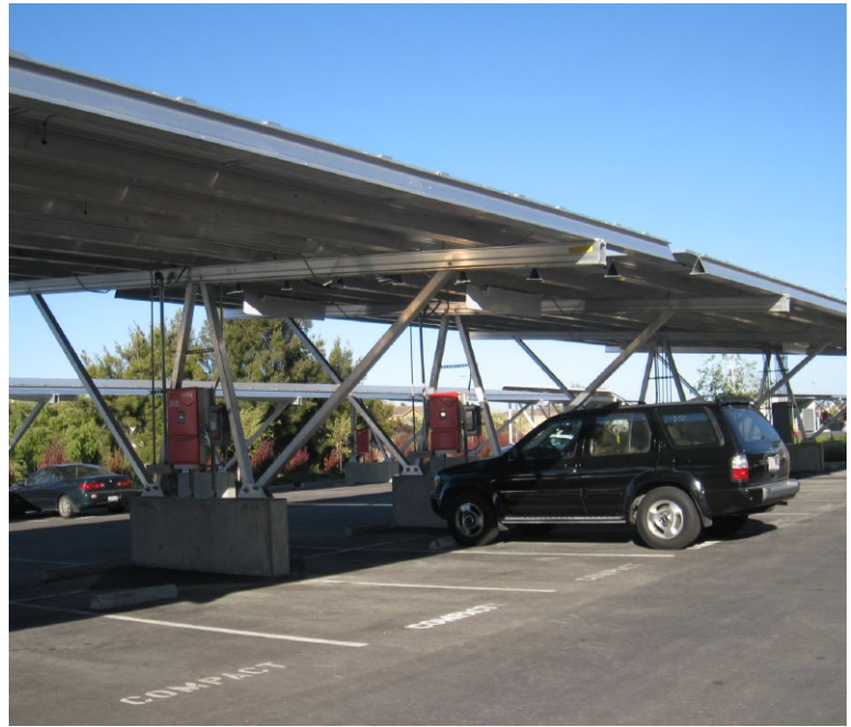
Solar panels serve as shade structures in parking lots
