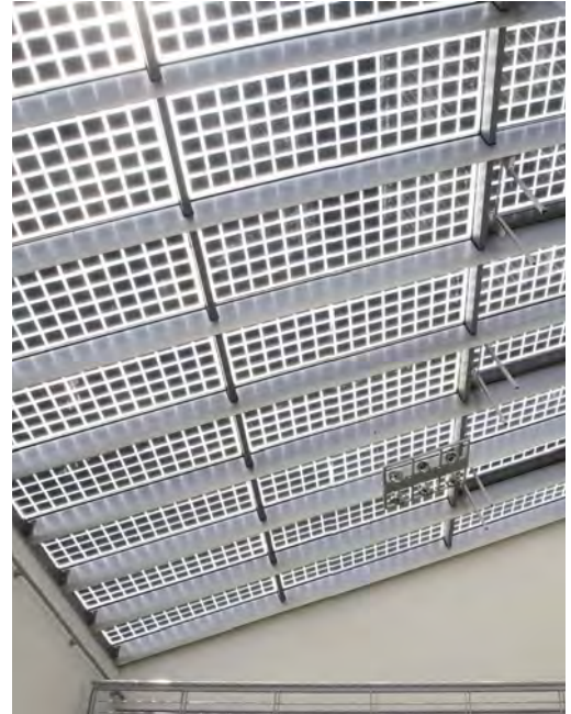
Solar panels integrated into glazing
