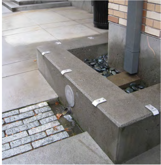
Downspout is directed under pavement into a rain garden
