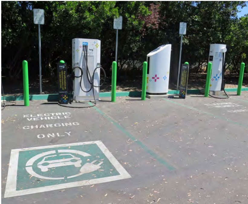
Electric vehicle parking and charging stations
