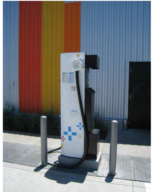
Electric vehicle charging station
