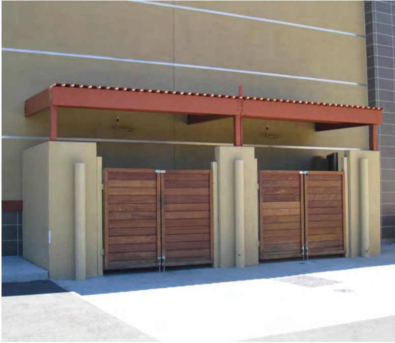
Recycling and garbage are located in the same enclosure, but separated from each other
