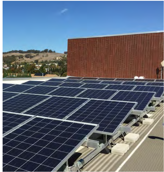
Brick tower element screens solar panels from the street
