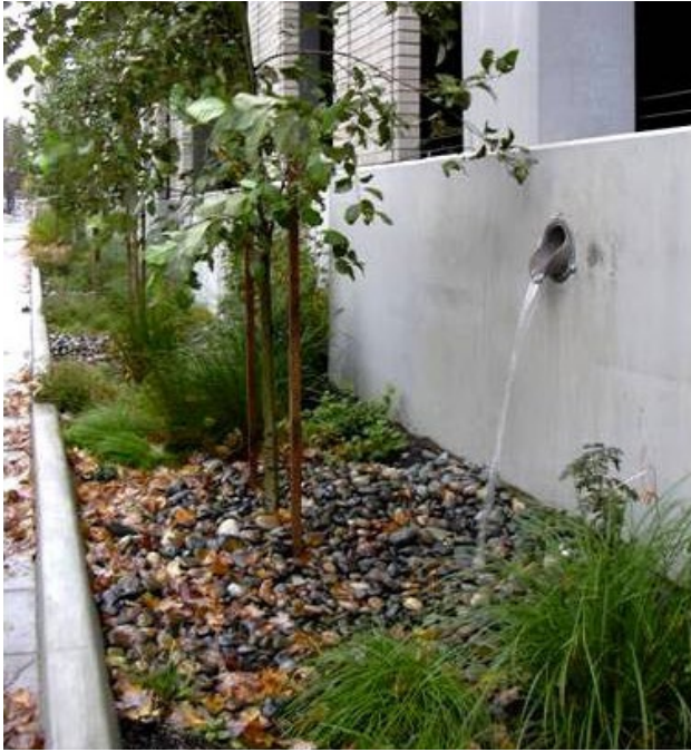
Roof downspout empties into planter
