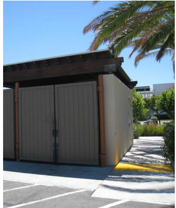
Clear pathway of access adjacent to enclosure
