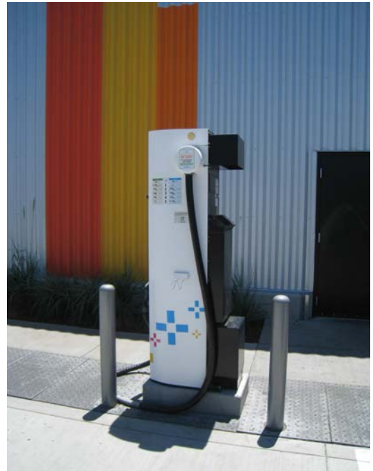
Electric vehicle charging station
