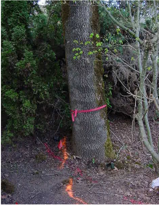
Tree is not properly protected from construction
